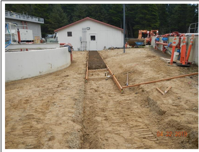
Surface grading and installing a gravel walking path to the FEB blower room.
