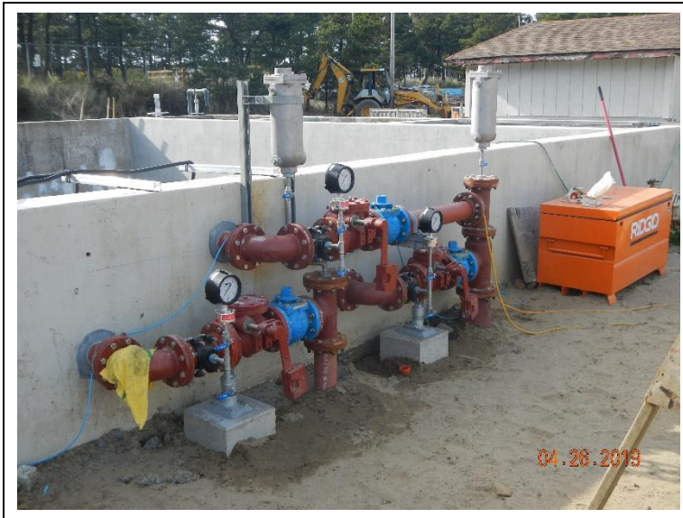
Installed air relief valves on the FHT pump piping.
