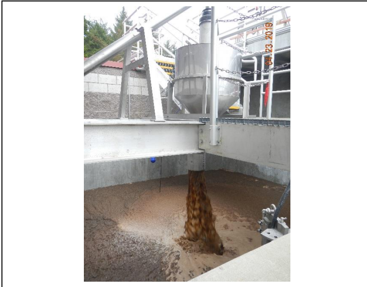
Lime stabilizing sludge in the lime tank.
