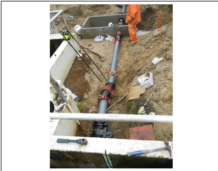
Installing the reuse water piping from the UV effluent channel to the valve vault.
