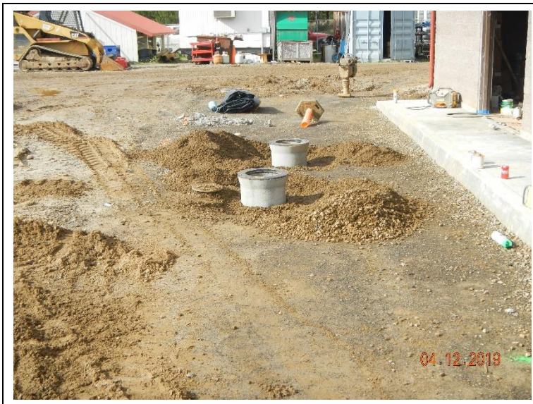
Setting valve covers and clean out covers along the SBR access road.
