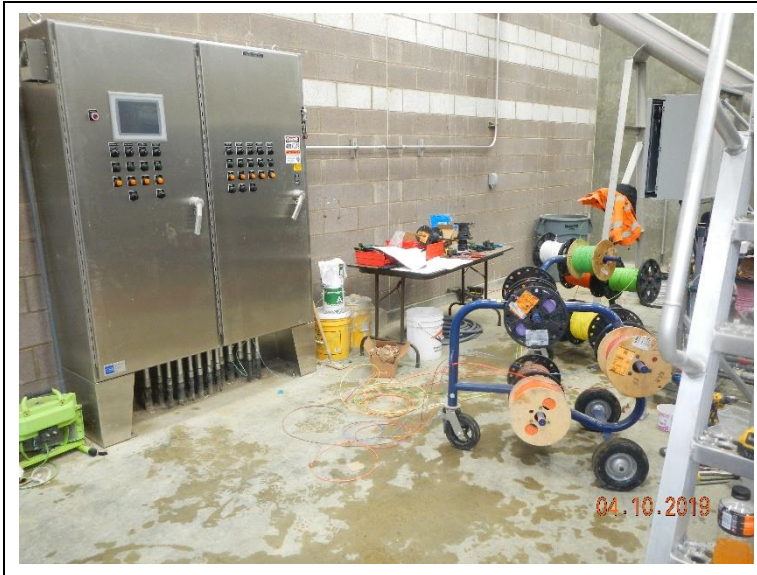
Preparing to pull wires from the solids control panel to the solids' equipment.
