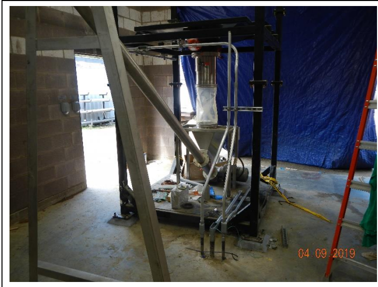
Installing electrical conduits to the lime discharge unit and conveyor in the lime room.
