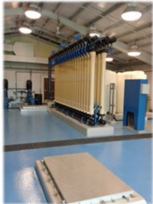
Horn Creek Microfiltration System
